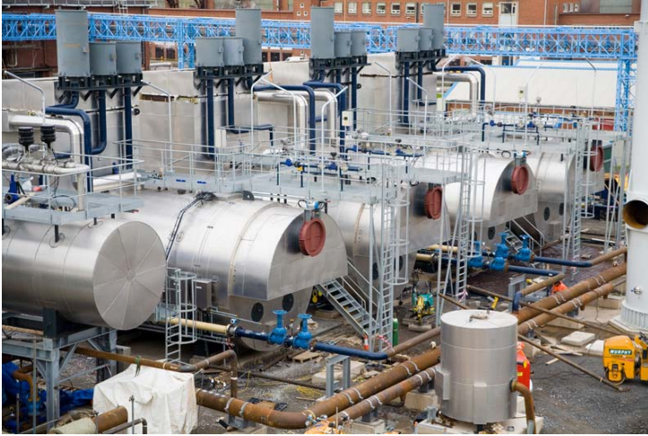
The four package boilers adjacent to Wilton Power Station
